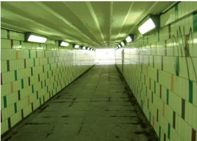
The southern underpass needs significant improvement to enhance the quality connection to the proposed secondary school at Bow Locks
